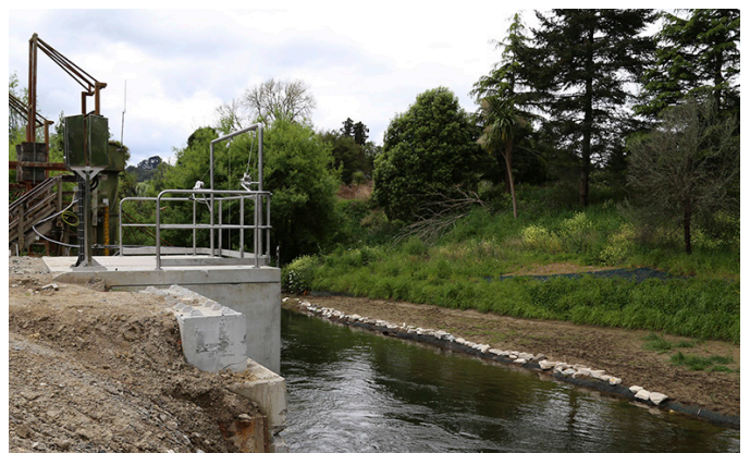
RIVER INTAKE AT TE KUITI WATER TREATMENT PLANT
