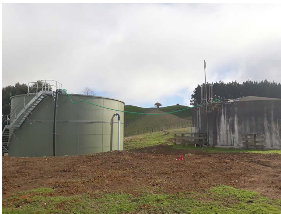
NEW PIOPIO WATER RESERVOIR (LEFT) AND OLD (RIGHT).
