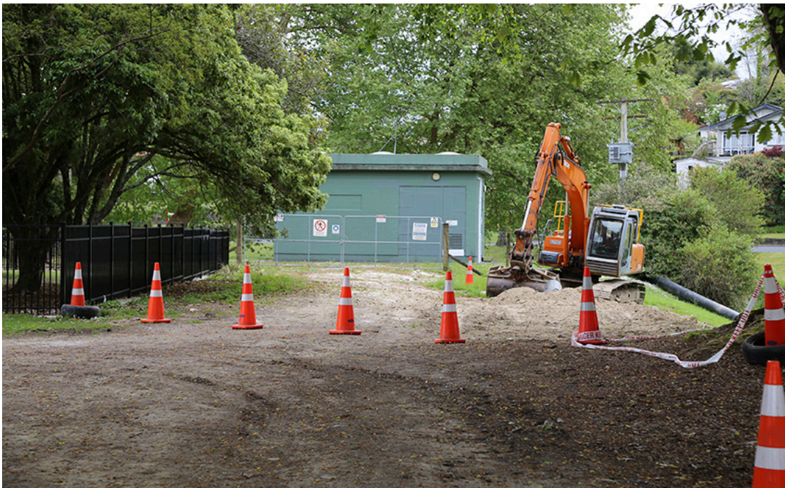
MAIN SEWER PUMP STATION TE KUITI
